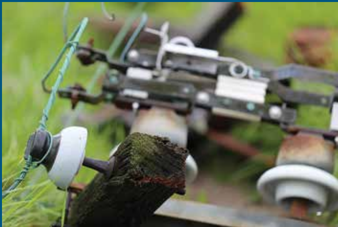
Top: Rick Mersinger, maintenance foreman; Braden Clark, journeyman lineman, and Jimmy Revisky (also at right), construction foreman, ready a pole for installation.
