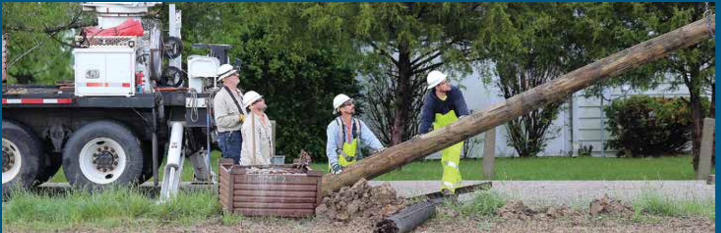
Top: Jake Cain, forestry journeyman (left), and Alex Goodin, forestry foreman, help Kari Wise of Marine detour around construction while Tyler Kunz, journeyman lineman, Prepares to connect power lines to a new pole. Above: Mersinger, Kunz, Revisky and Clark guide a pole into position. Below: Crews make final repairs before energizing lines on Rockwell Road in Madison County.
